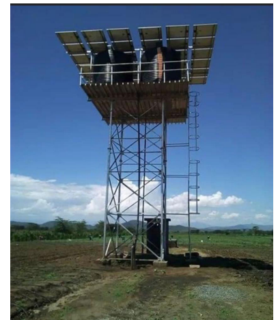
Kuresoi health centre borehole Elevated tank tower
