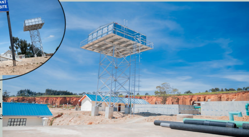
A section of Olkalou Water Treatment Plant
