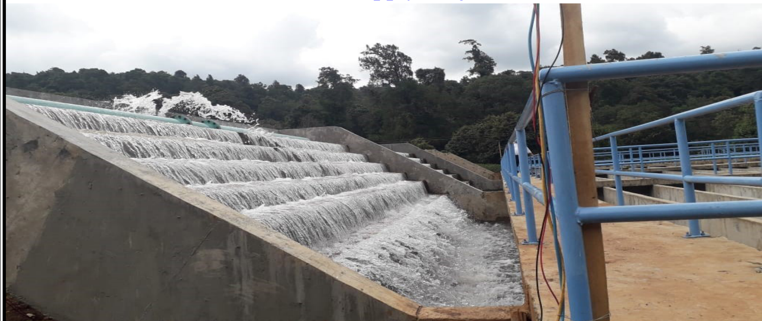
A section of Chemususu Phase II Water Treatment Plant.
