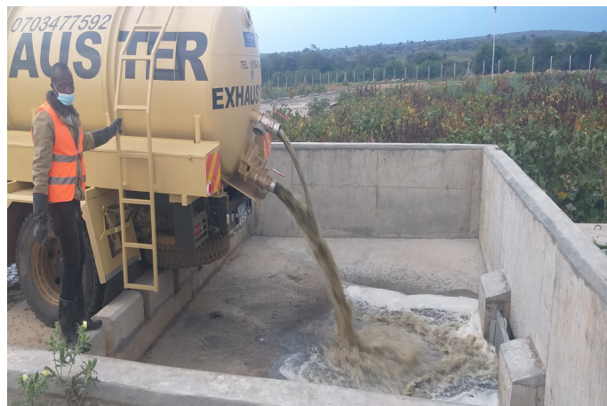
Exhaust discharge bay
